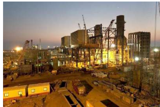
Figure 6 Reliance Power Plants
