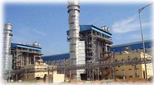
Figure 7 Gas Turbine Power Plant of ONGC
